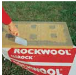
— Applying Kale Mantotech Thermal Insulation Board Adhesive Mortar along the edges of the boards.
